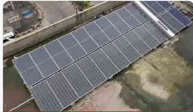
50KW rooftop PV project in Jakarta, Indonesia
