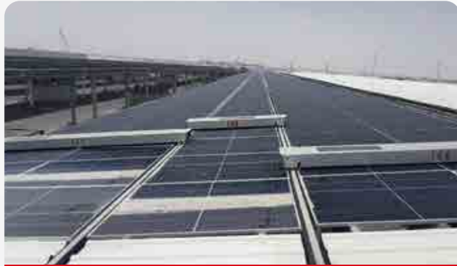
6.3MW Qatar World Cup-Transportation photovoltaic power station
