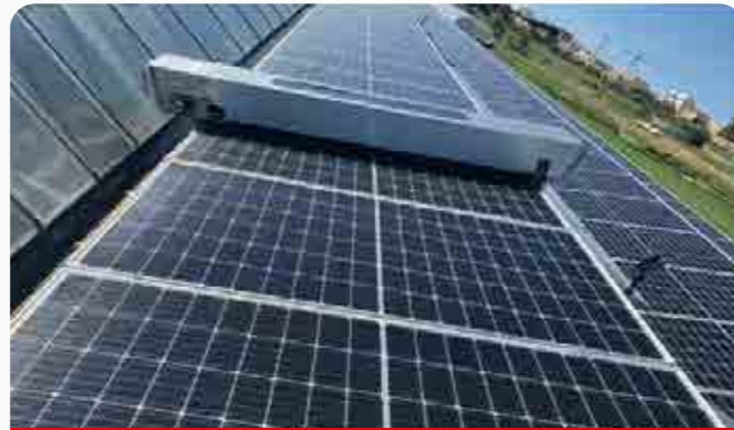
5MW ground PV power station in Maltese
