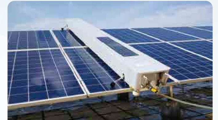
200KW PV poverty alleviation power station in Zhengzhou, Henan province
