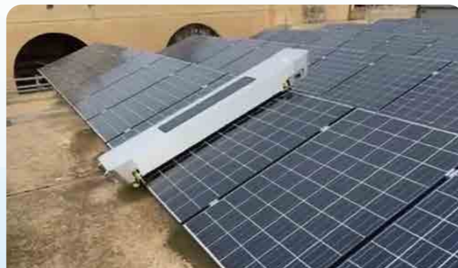
1.5MW rooftop PV power station in Turkey
