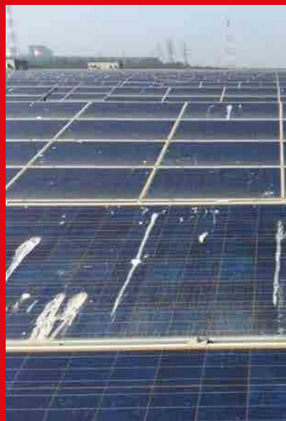
① Pollutant Rust
