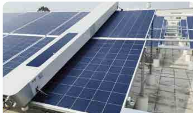
200KW rooftop PV power station bridge in Guang'ao, Shantou
