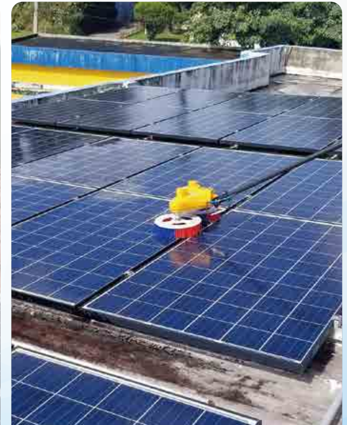
5KW Roof in Puerto Rico
