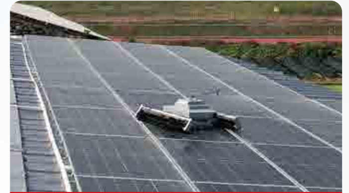
25.5KW rooftop in Hebei
