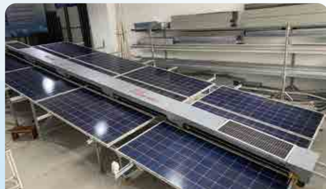
50KW in Belgium
