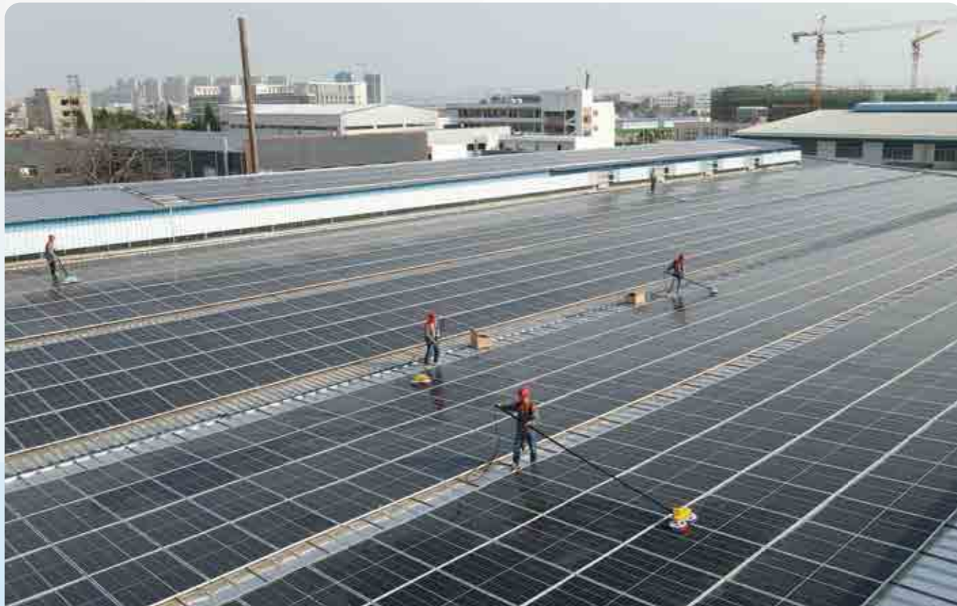
114KW solar plant in Chaozhou
