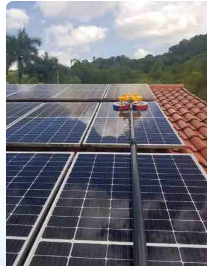
3KW Roof in Thailand
